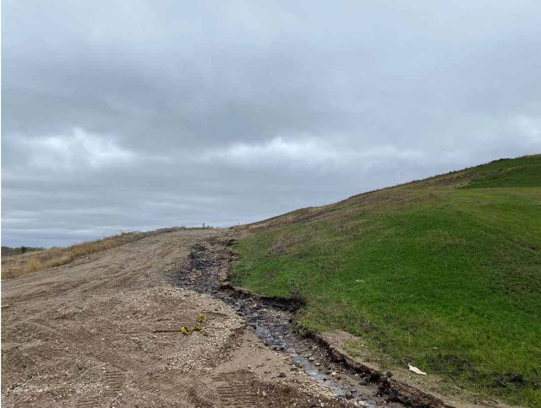
Location 3 – Looking Southwest, Cell 3 East Corner at toe of Interior Access Road
